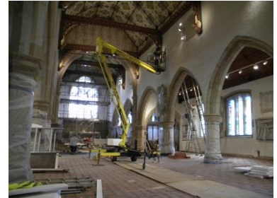
Cherry pickers permissible to 2 tonnes with additional layer of 2 x 18mm ply.
