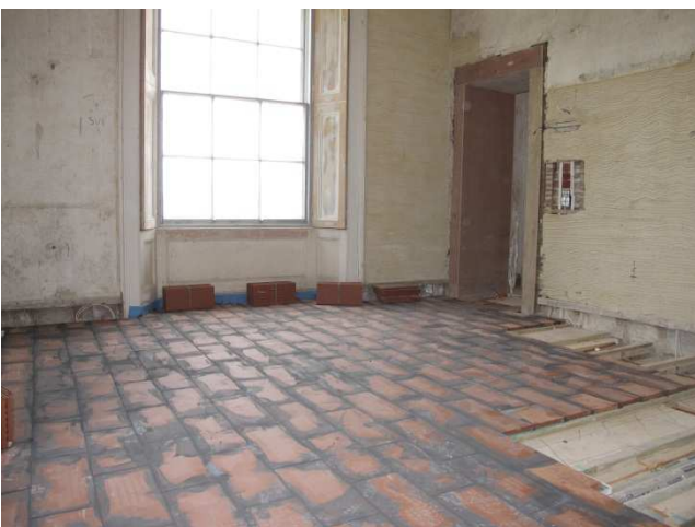
As all bathrooms were to have stone floors the Screed Replacement Tile was specified to provide high heat output and a stable substrate.
