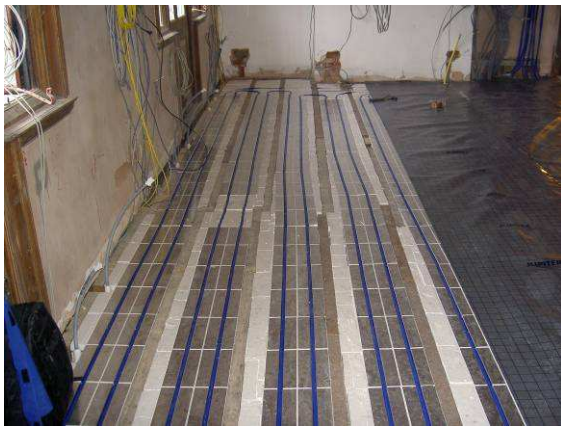
IDEAL System installed within existing joists. Resting on additional insulation resting on battens and ply supporting sheets.
