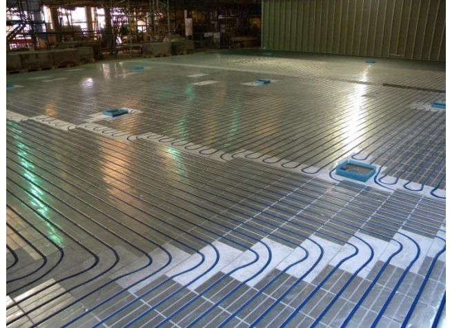
Installation of Ideal EPS heating panels with 125mm pipe centres providing maximum output and allowing for floor boxes within the floor
