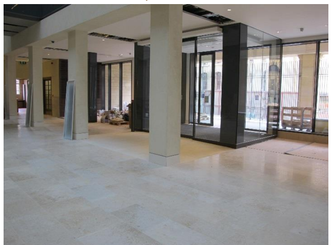
The finished result – an efficient and responsive underfloor heating system which guarantees that the finished floor will not fail
