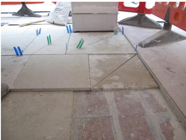
The limestone finished floor is installed on a full bed of adhesive with very few movement joints and no decoupling membrane due to the inert nature of the SRT substrate
