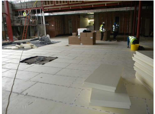
With previous experience of the JUPITER product range and a very tight program the contractor elected to use the IDEAL EPS system with the Screed Replacement Tile as substrate.
