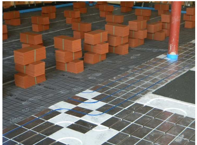
Installation of the 465m² Screed Replacement Tiles took just under two weeks – drying time 1 day.
