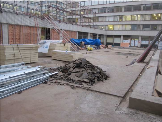
What was originally an external courtyard was to be transformed into a new outpatient centre.
