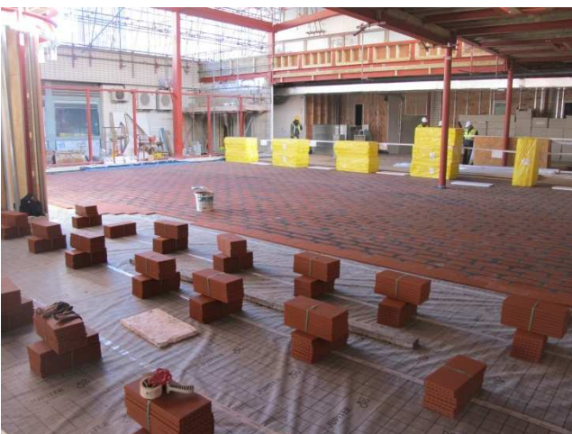
Once installed, the Screed Replacement Tiles were levelled with a latex compound in readiness to accept the vinyl floor finish.
