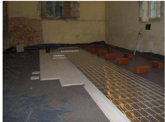
For maximum output a total area of 150 m 2 of IDEAL EPS Edge Zone panels were used. These panels have the pipes positioned at 125mm centres.
