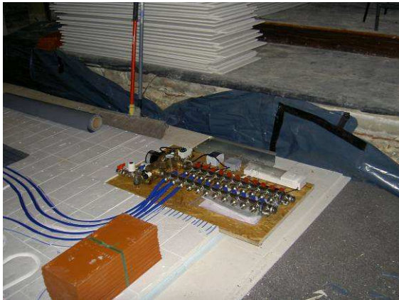
As with previous projects the underfloor heating manifold, mixing valve and pump were installed flat on the floor in order to be housed centrally in the church under the Deus.
