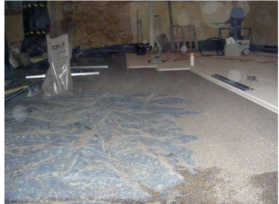
The void left by the removal of the existing floor was filled with recycled foamed glass which replaced traditional hardcore and concrete. The foamed glass also provides additional insulation.
