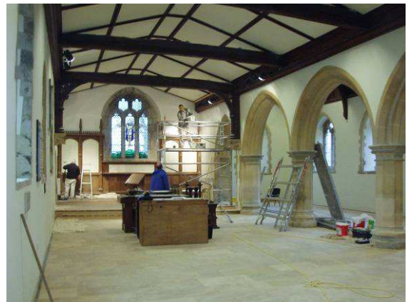
The large format natural stone floor slabs are then adhered flexible tile adhesive to the Screed Replacement Tile system without the need for any movement joints or decoupling system.
