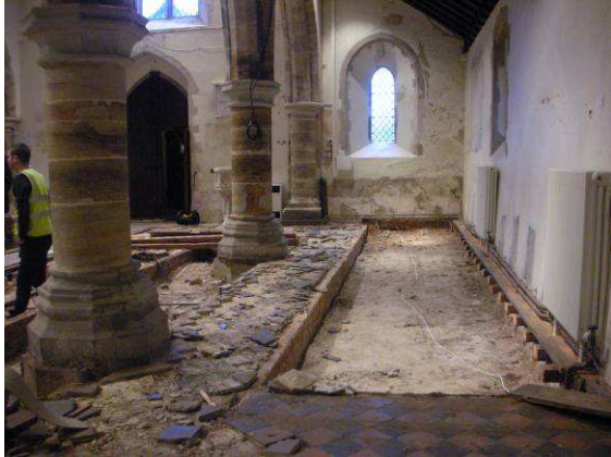
The existing Victorian floor was removed in collaboration with Sussex Archaeology. Finds were recorded and exposed vaults bridged with a beam and block construction.
