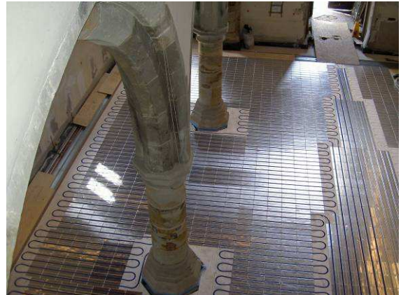
For maximum output a total area of 141 m 2 of IDEAL EPS Edge Zone panels were used.
