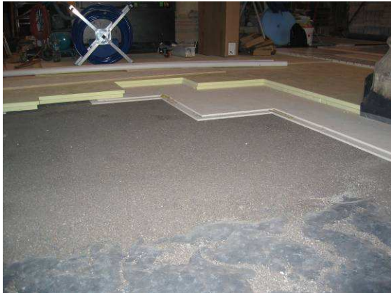
A DPM was laid over the foamed glass and then levelled with granulated slate which was in turn covered with Fermacell flooring elements. High density Collecta XPS insulation was then installed prior to the JUPITER IDEAL EPS system being installed.
