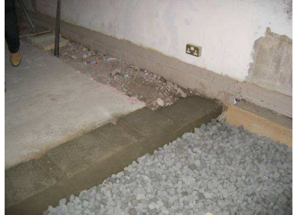
The main void left by the removal of the existing floor was filled with recycled foamed glass which replaced traditional hardcore and concrete. The foamed glass also provided additional insulation.
