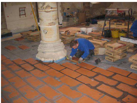
The JUPITER Screed Replacement Tile is finally installed over the IDEAL heating system as the final substrate to the floor finish
