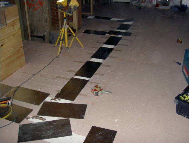
Installation of Kingspan K3 with in filled service channel covered with steel sheet
